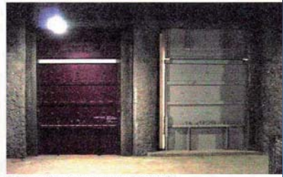
粘性体制振壁 (六本木ヒルズレジデンスB・C棟) Seismic Damping Walls with viscous core (Residences B and C)
